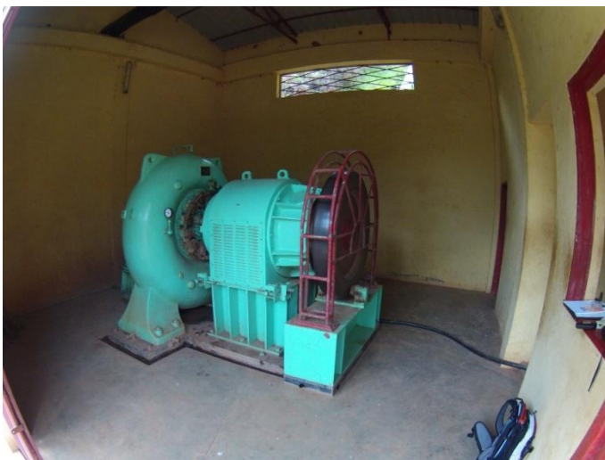
turbine and generator
