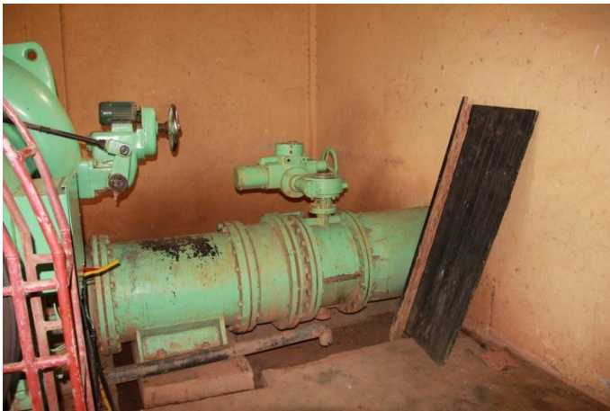
penstock inside ph, DA 720 mm
